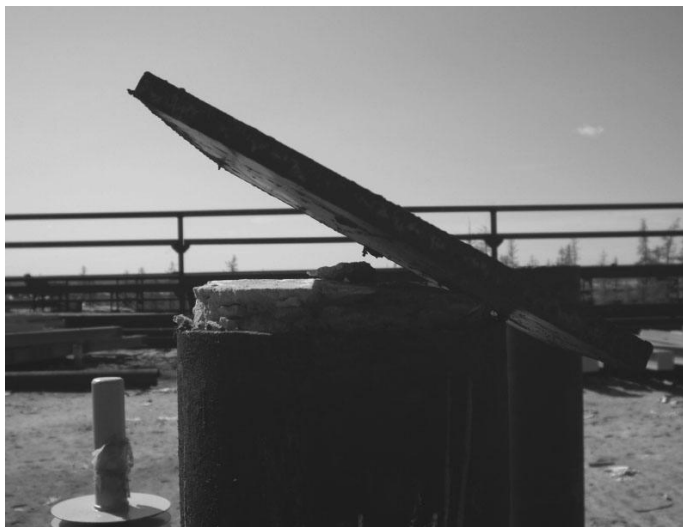
Figure 2. The uplifting of the pile head due to heaving of the sand and cement mortar inside the pile with the diameter of 159 mm.
