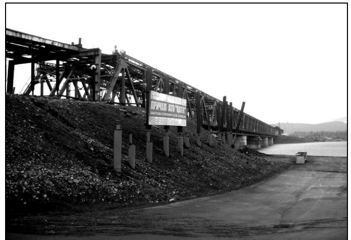
Fig. 1. Deformed motor- and rail-road bridge across Norilskaya River, with deeply embedded vapor-liquid thermal units along the left pile contour (Photograph by A. Maslakov, July 2010).
