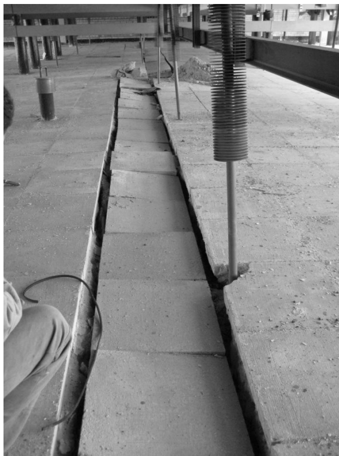
Figure 3. Ground cracking along the longitudinal axis in the vented crawl space.
