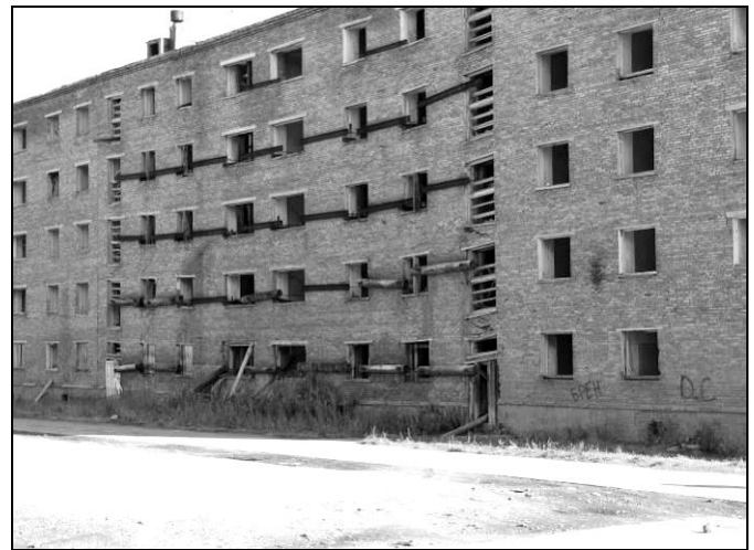
Figure 1. Activities aimed at preventing deformations of a residential building in the 1st district. The central part of the building is dragging the side parts along. (Photo by S.V. Poznarkova, July 2010).
