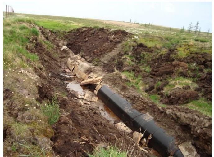
Figure 1. Thermal erosion at the construction site of the underground gas pipeline at the Yamsovey Field, the north of Western Siberia. July 2009. The photo by V. Grebenets
