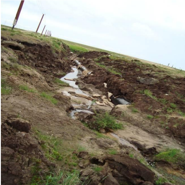
Figure 1. Exposure of the underground gas pipeline at the Yubileynoe gas field area in the process of thermal erosion development, July 2009.
