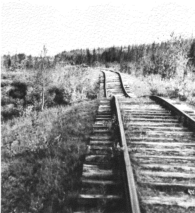
FIGURE 1 Settlement of a roadbed caused by thawing of the permafrost in the subgrade (photograph by the author).
