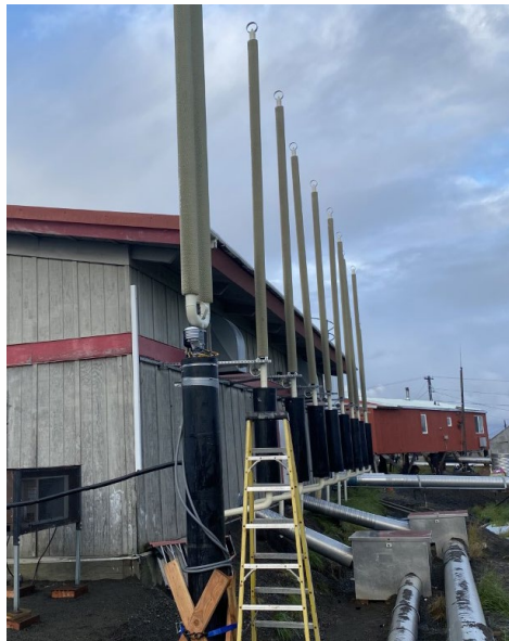
Upgraded thermosyphons at the Water Treatment Plant, Quinhagak, AK.
