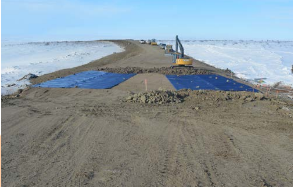
Fig. 11. Wicking geotextiles laid during construction of a reinforced section of the ITH.
