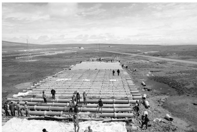
Experimental expressway section at the Beilu'he Permafrost Station in the interior QTP under construction. The four-layer air-ducts were used for stabilizing warm and ice-rich permafrost foundations. (Photograph provided by Qihao Yu)
