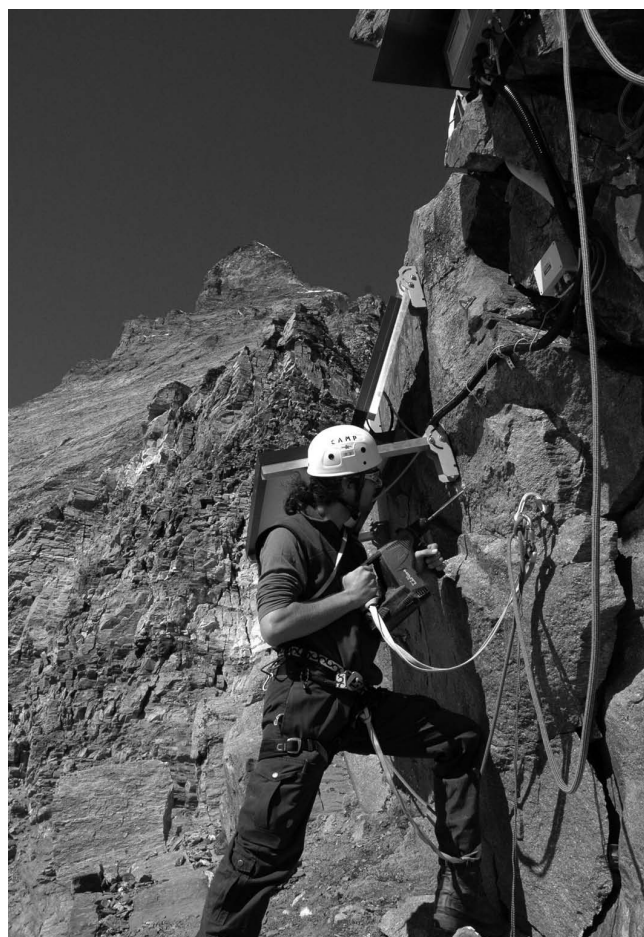
Sensor installation with Matterhorn in the background. Permasense wireless network. (Photograph provided by Jan Beutel)
