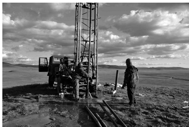
Drilling in sub-pingo water layer at 32.4m depth at the top of Mongot pingo, August 8, 2009. (Photograph provided by Kenji Yoshikawa)
