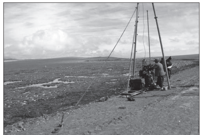
for the installation of monitoring boreholes along the railway route from Muli to Reshui in the Qilian Mountains.
